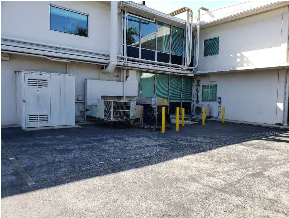
Photograph 2 - View of electrical transformers and air conditioning units adjacent to Building 2. Note cleanliness of area and placement of protective bollards.
