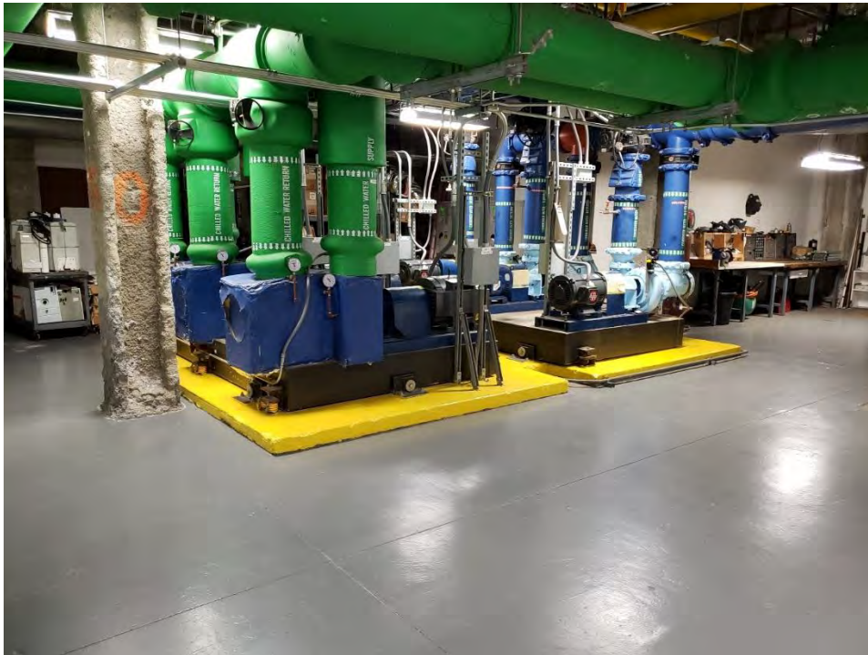
Photograph 10 - View of machine/maintenance area within basement area of Building 15. Note well-maintained equipment and cleanliness of surrounding areas.
