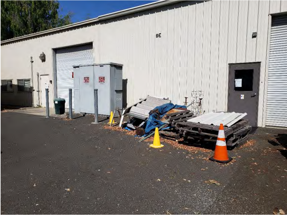
Photograph 4 - View of debris pile adjacent to transformer on east side of Building 9E.
