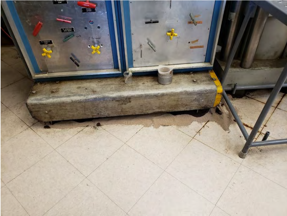
Photograph 7 - View of contained fluid leak beneath industrial machinery within Building 10. Note absorbent material used to keep leak within machine footprint.
