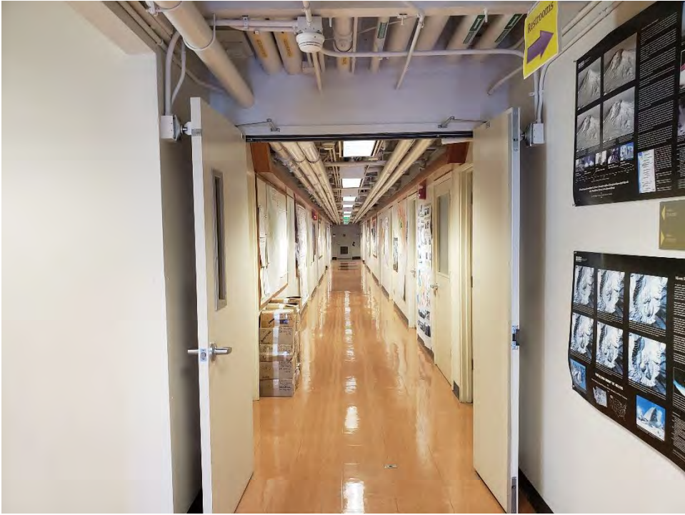
Photograph 3 - View of interior hallway of Building 2. Note exposed but well-maintained ceiling piping.
