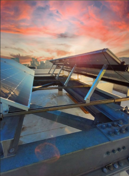
Figure 11. Solar on U.S. Constitution of Transportation, Ridge Center, Cambridge, MA
