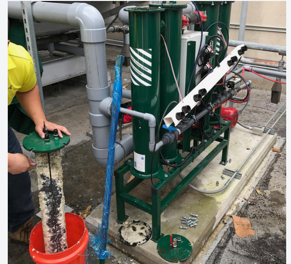
Scraping scale off the reactor rod of the electrochemical water treatment system. Photo credit Gregg Tomberlin, NREL
