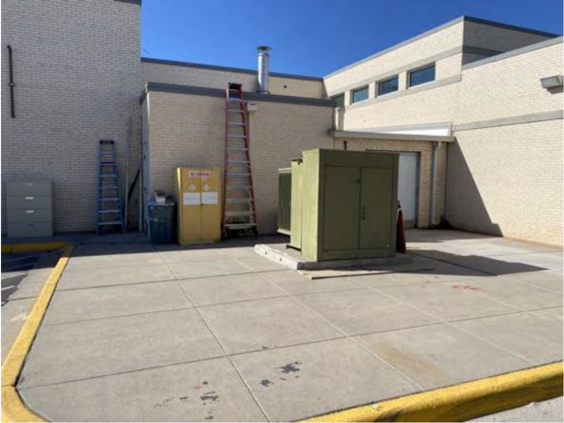
Photograph 29: View looking west of the pad-mounted transformer near the admin building.
