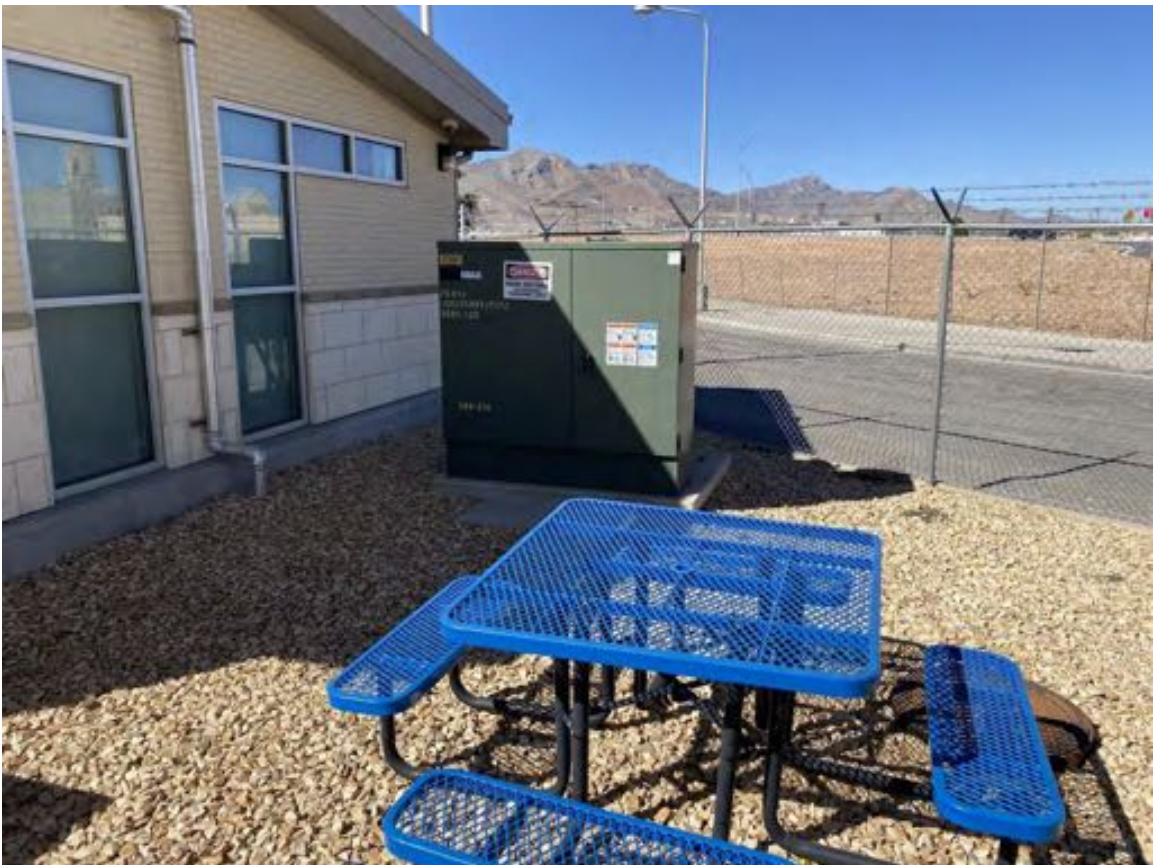
Photograph 28: View looking northwest of the pad-mounted transformer on the northern end of the POE property.
