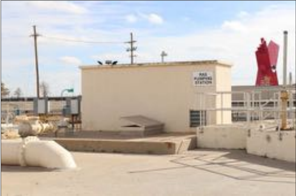
Figure 264. RAS Pumping Station, looking south.
