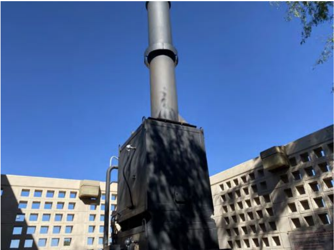
Photograph 32: View looking north of the incinerator near the admin building.
