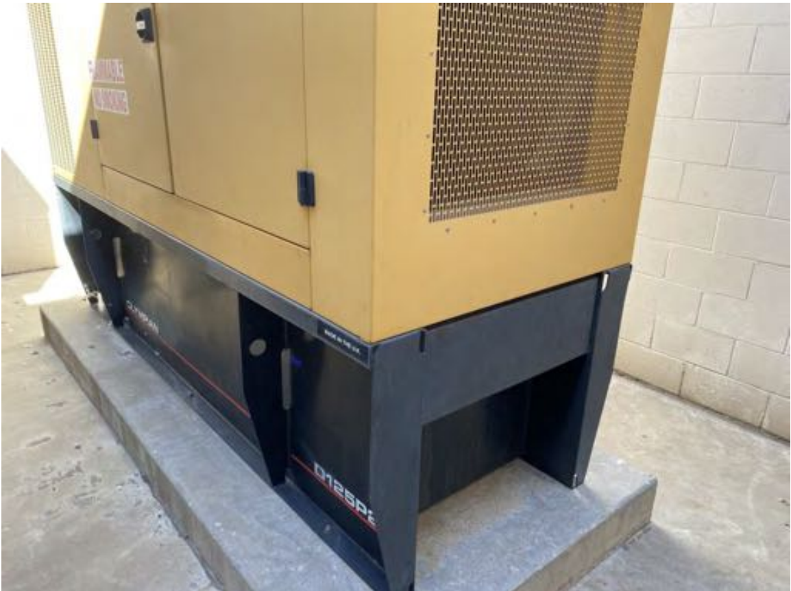
Photograph 26: View looking northeast of the emergency generator and belly fuel tank located in the secondary vehicle inspection area.
