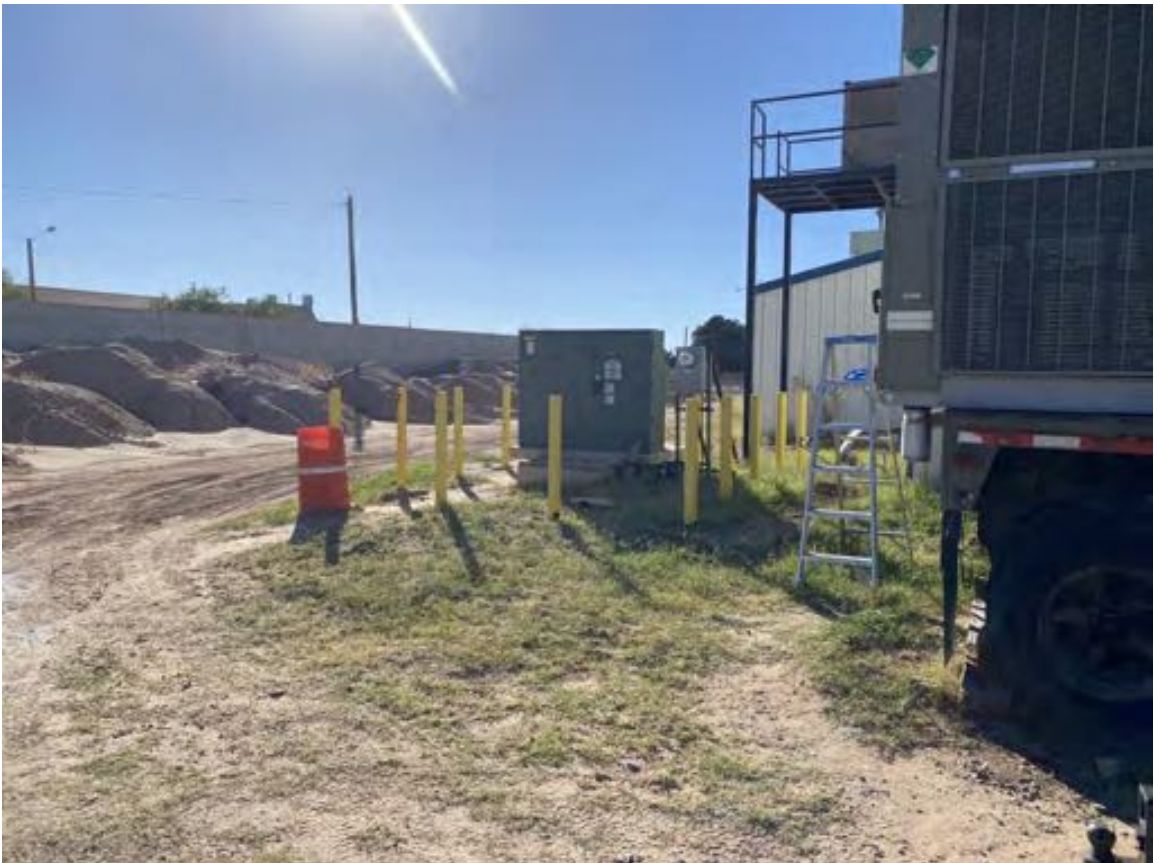
Photograph 30: View looking west of another pad-mounted transformer south of the County events center/hockey rink.
