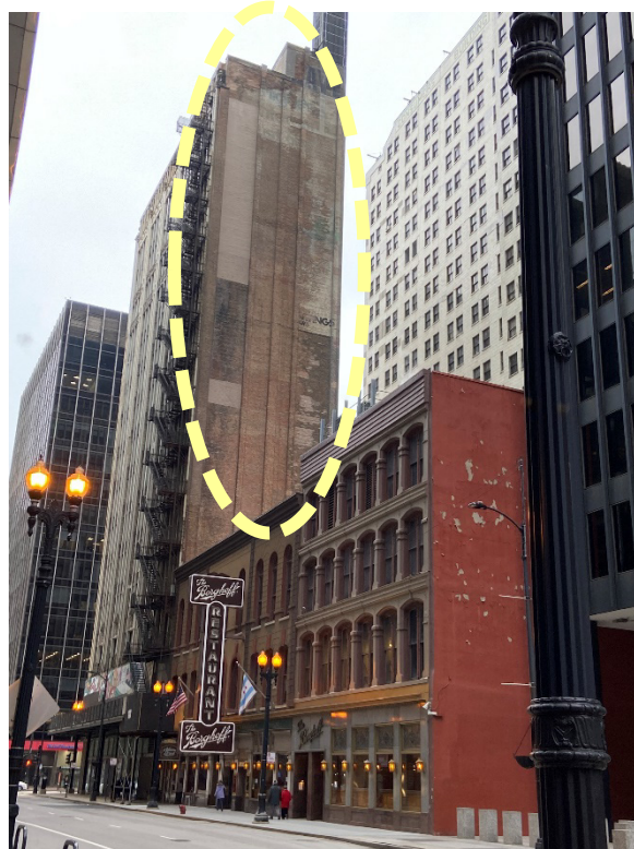
Figure 3.2-4. Picture Taken on Adams Street showing West Elevation/Face of 202 South State Street (circled). Fire escape since removed.
