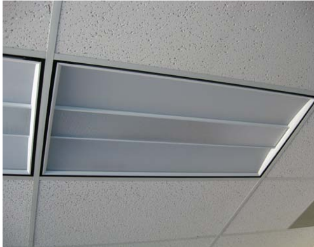
Figure 114: Example of two-lamp 2x4 recessed troffer lighting fixture with lens
