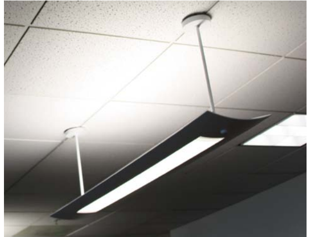
Figure 115: Example of three-lamp pendant fixture
