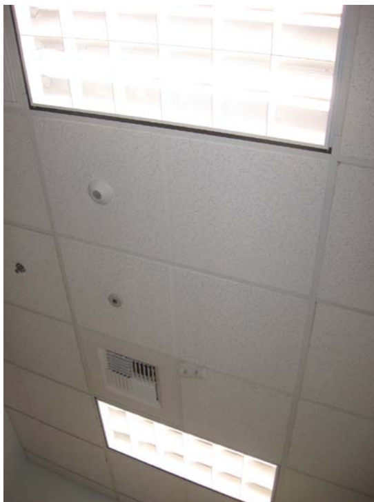
Figure 116: Example of two-lamp 2x4 recessed troffer lighting fixture without a lens
