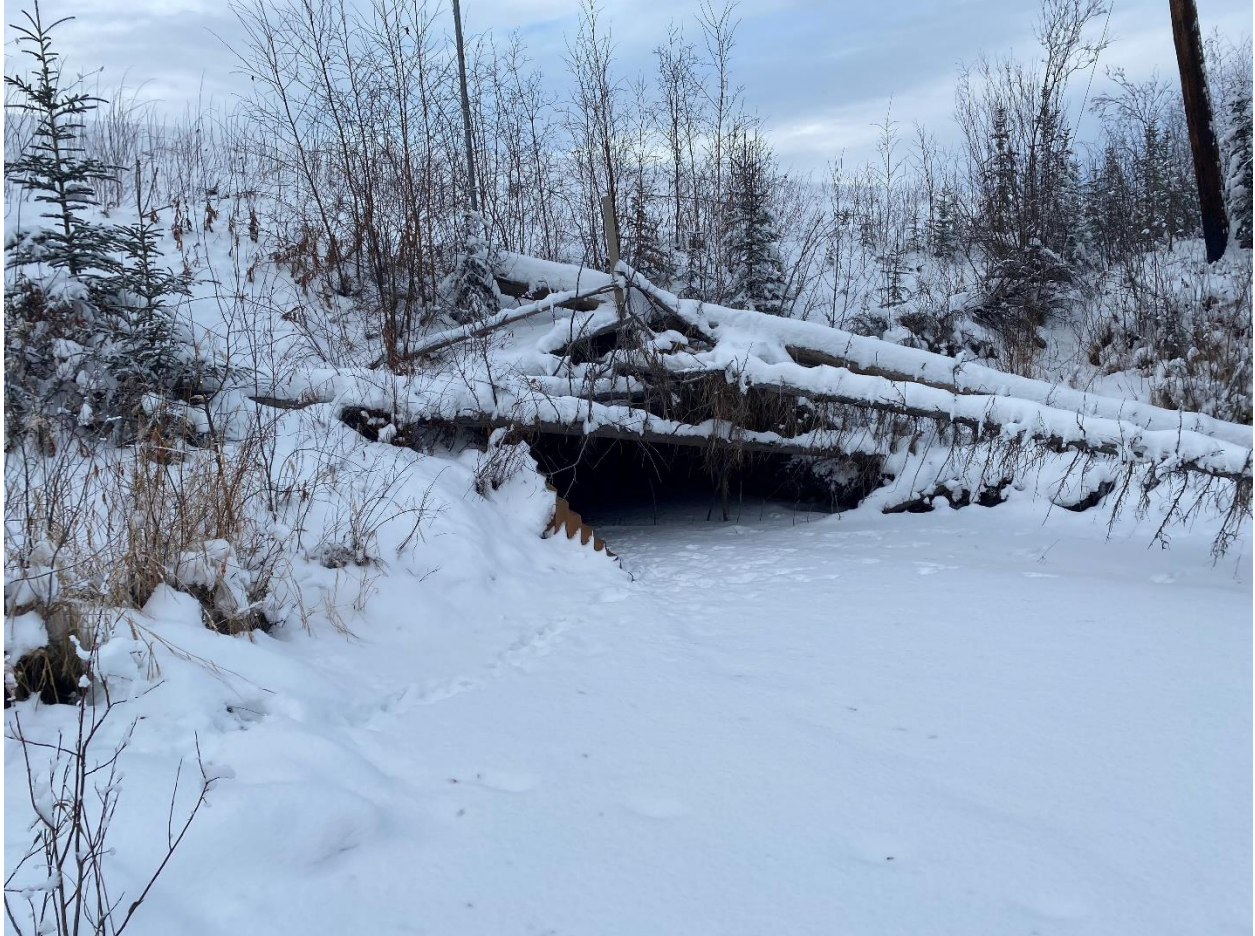
Figure 6. Bridge No. 7084 (culvert) at Desper Creek with woody material blocking upstream opening
