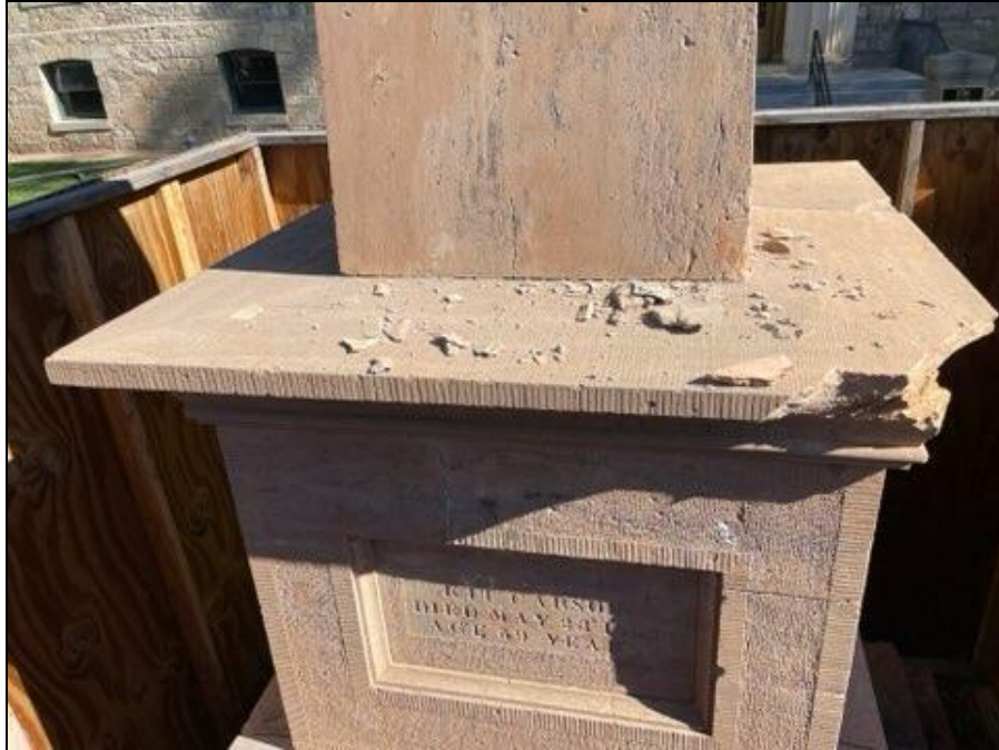
Figure 12. Kit Carson monument, damage to the cornice (photo taken September 2023).
