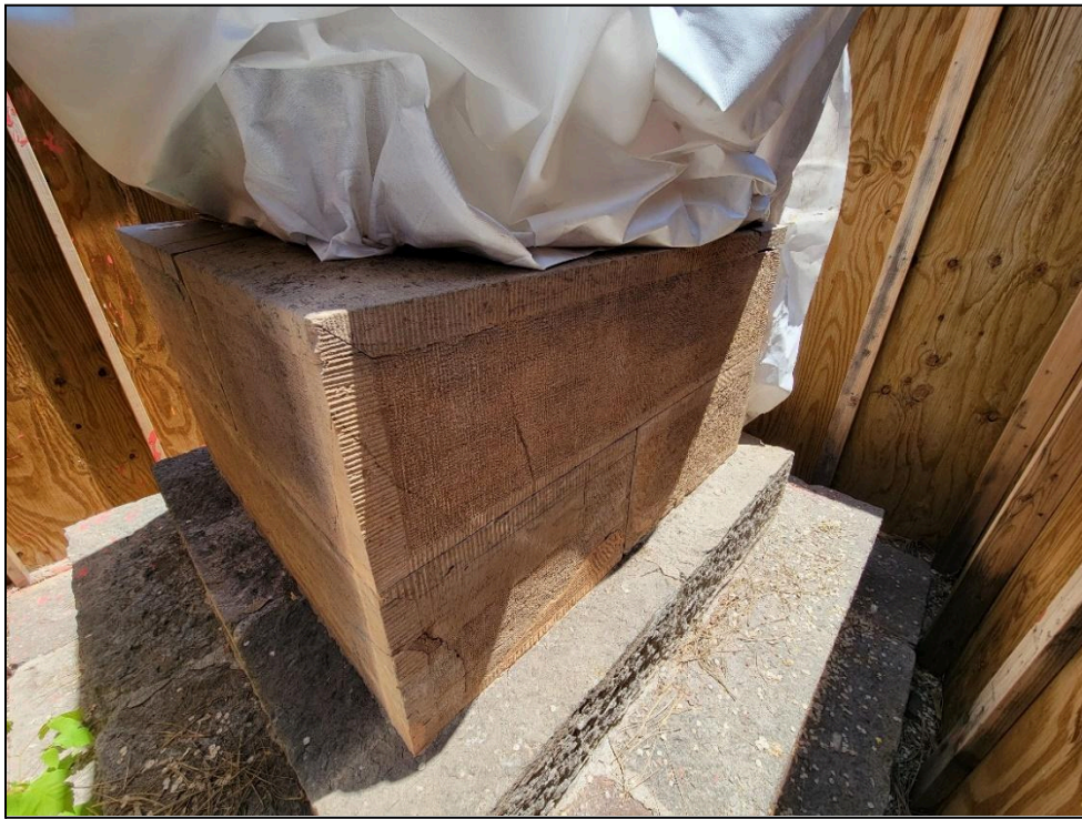
Figure 17. Kit Carson monument, view of steps and base (photo taken June 2024). Note cracks in base.
