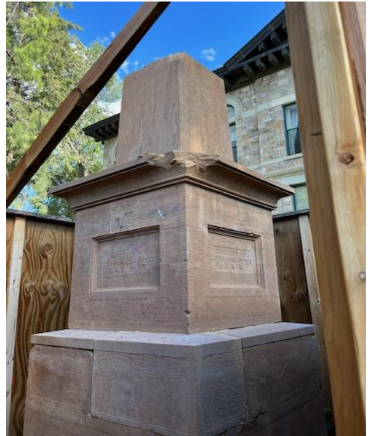
Current condition of monument within the plywood box. The monument has lost most of its height.
