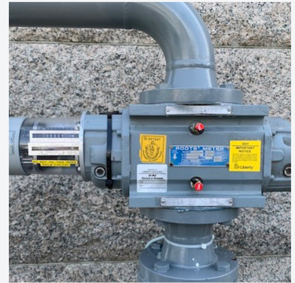
Non-Invasive Gas Submeter Photo credit Vata Verks
