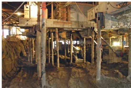
Interior view of the base isolation system being installed at the Pioneer Courthouse.
