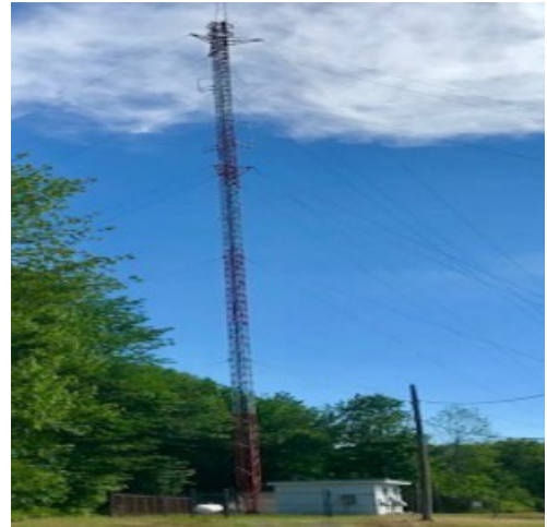
Photograph STR-2: This photograph is an example of an antenna tower which holds multiple antennas.
