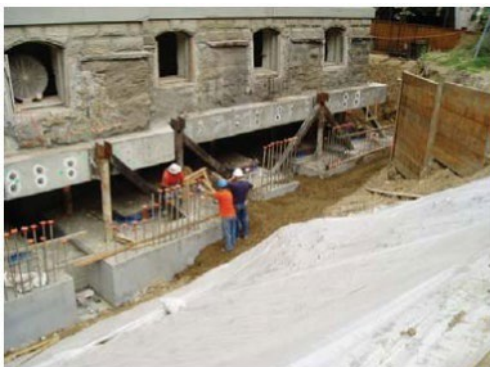
Exterior view of the Pioneer Courthouse being retrofitted with a base isolation system.
