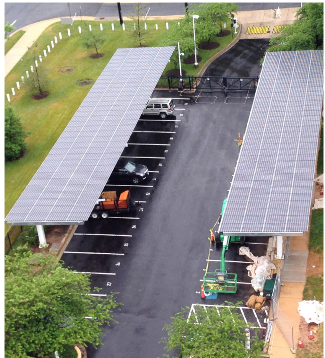
South parking lot PV canopy Image courtesy of: Ameresco, Inc.
