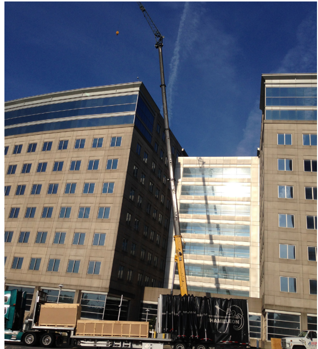
Heat recovery coil installation Image courtesy of: Ameresco, Inc.
